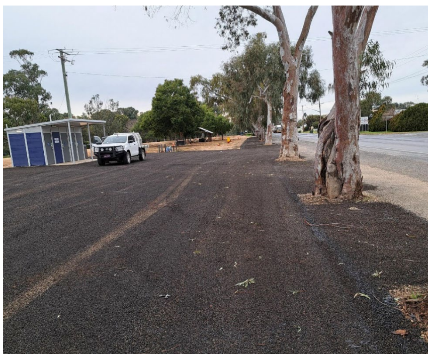
Figure 3: The toilet and barbeque area at Rotary Park was sealed in July. Lawn is to be installed around the shelter
